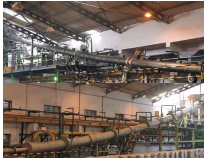
Figure 1 : 6 Nos. CCV (DRY CURE) LINES
